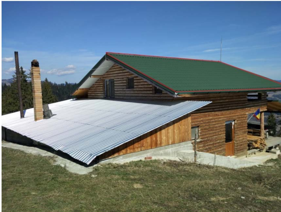
Figure 23: Installation place of the solar panels. Source: Own
