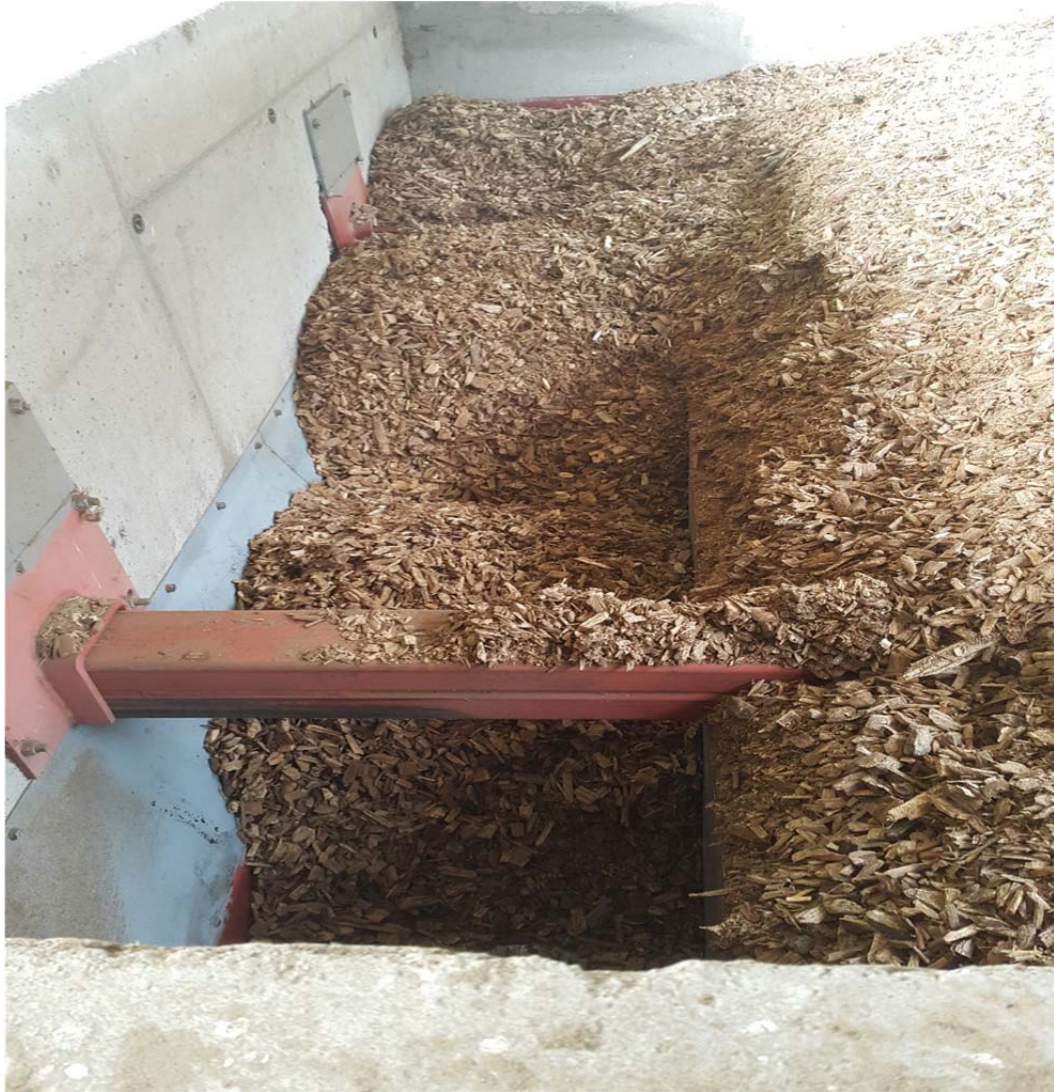
Fig.19. Storage bin and fuel handling system
