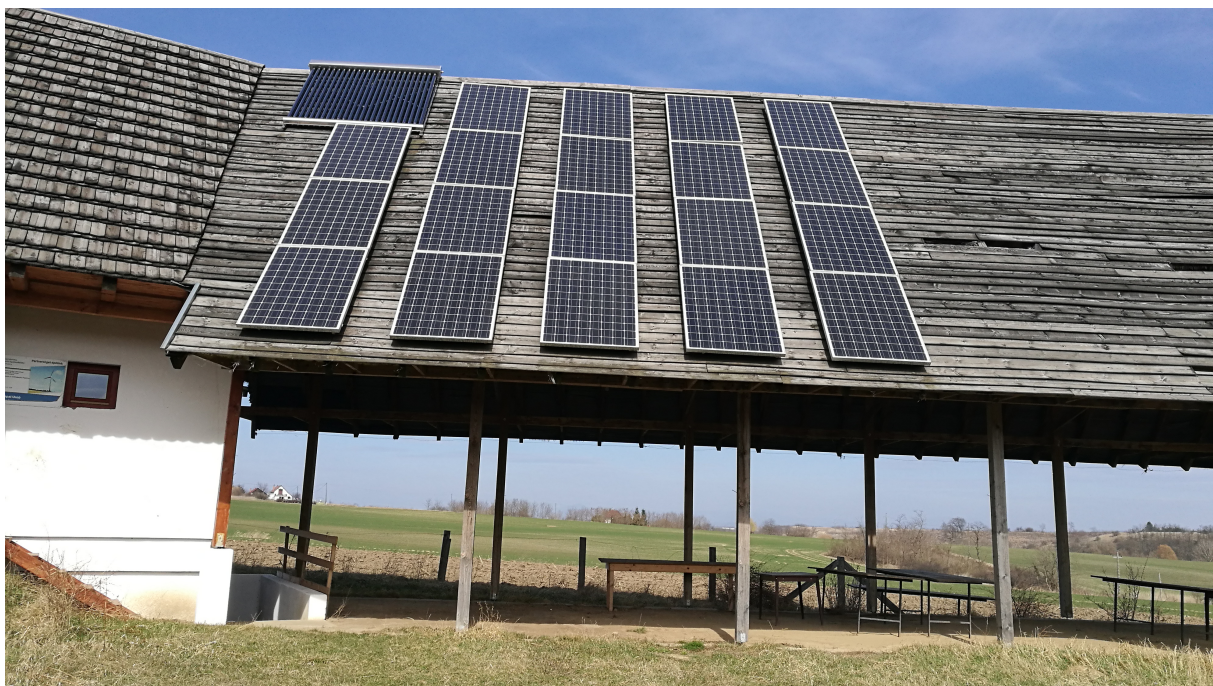
Figure 5- Photograph of a portion of installed solar panels
