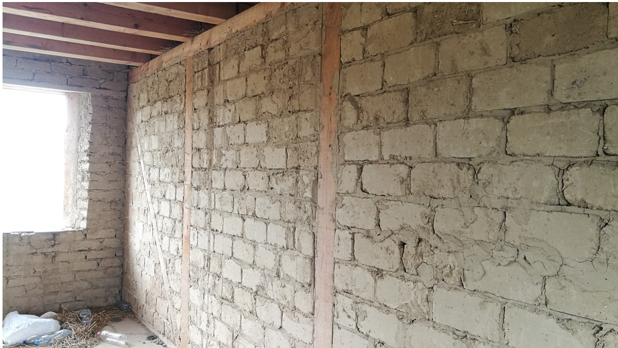
Figure 10 - Photograph of the wall inside the homes
