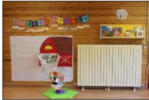
Figure 66. Radiator in the nursery. Source: Own elaboration
